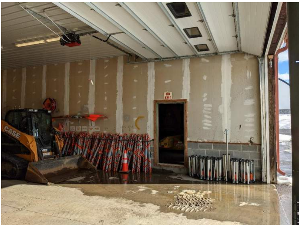
Facing east in equipment room.
