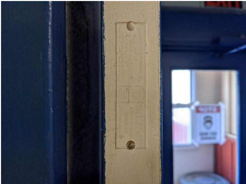
Fire door at entrance of Boiler Room.
