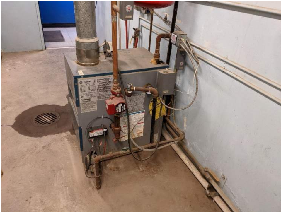
Boiler located in Boiler Room.
